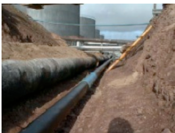
PROCESS PLANT, REFINERY AND LOCAL DISTRIBUTION PIPELINES
