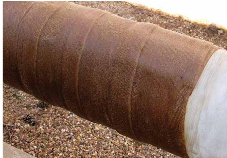
After coating with primer, the tape should be wrapped onto the pipe in a spiral pattering using a minimum 1" overlap. Seams and ends should be sealed.
